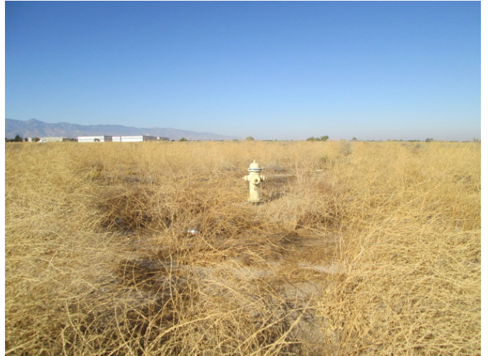
View of representative hydrant
